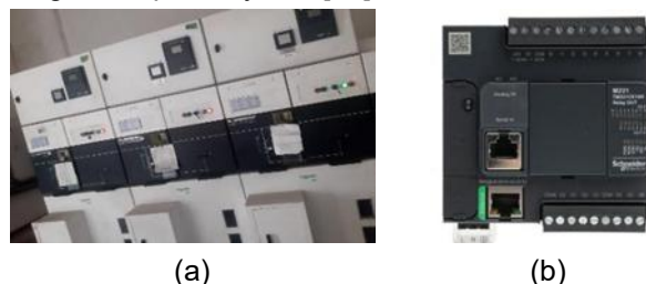
FIGURE 1. (a) Medium Voltage Cubicles, (b) PLC Schneider
